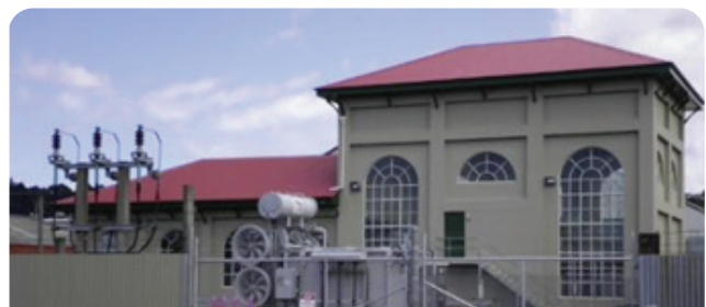
24 MVA 33/11/6.6 kV at Ward Street Substation, a heritage Substation building in Dunedin NZ
